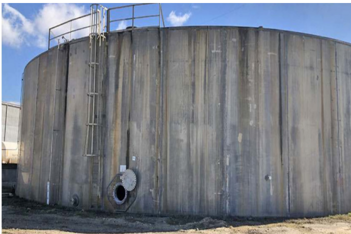
A huge fertilizer tank is slated to be redeveloped into an office building.
