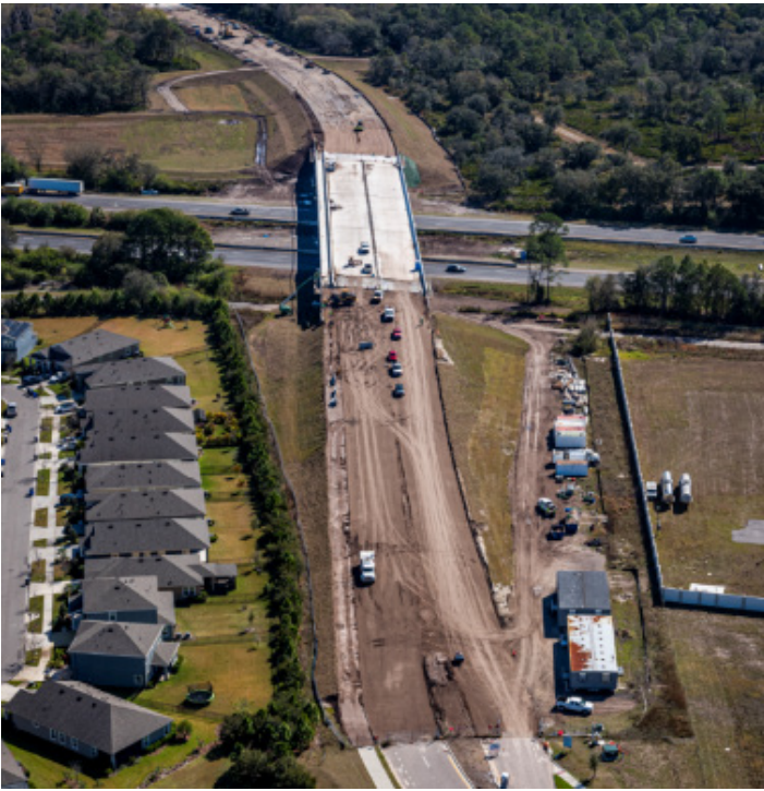
The Apollo Beach Blvd. (Paseo Al Mar Blvd.) I-75 Overpass provides connectivity between US 41 and US 301 - a vital east/west corridor in the South Hillsborough County area.
