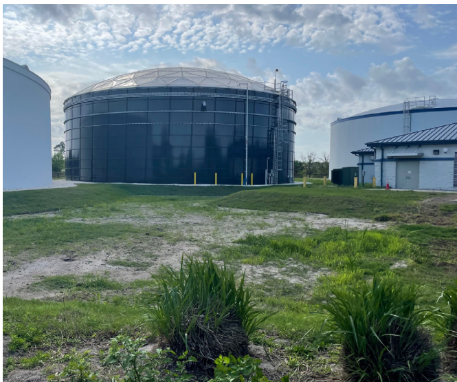
Tanks are shown at the South County Repump facility.
